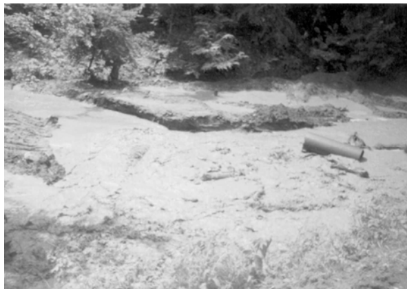
Fig. 2. A fragment of destruction by a flood in 2006 of a coastal zone of the river Agstev at village Agarcin
