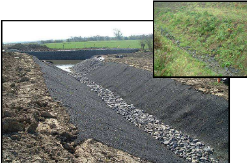
Photo 3. Insuring the stability of an irrigation-purpose main-line canal by means of “Sekumat”
