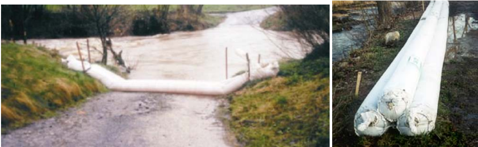
Fig. 4. Twin bag (filled by water), preventing water penetration from the ford and triple bag; (Terlicko, Stonavka River)
