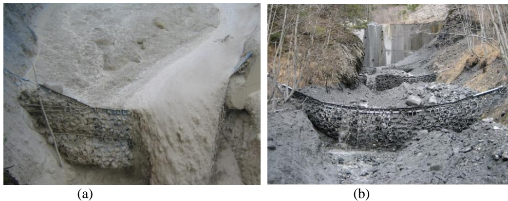
Fig. 2. (a): flexible ring net barrier withstanding overflow in the Illgraben; (b): 1:1 field testing of multi-level barriers in Merdenson, Valais, Switzerland
