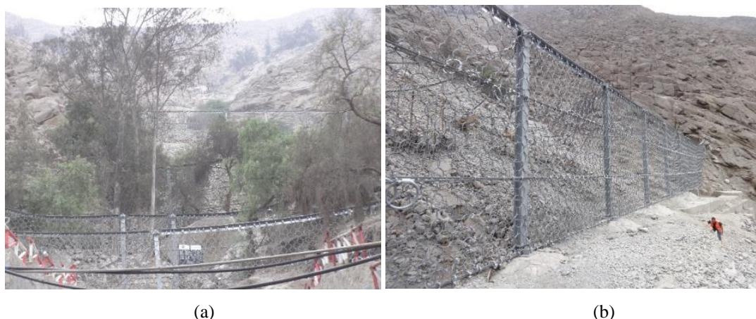
Fig. 8. Multi-level installation of flexible ring net barriers (left). The highest barrier is the largest in South America (right)
