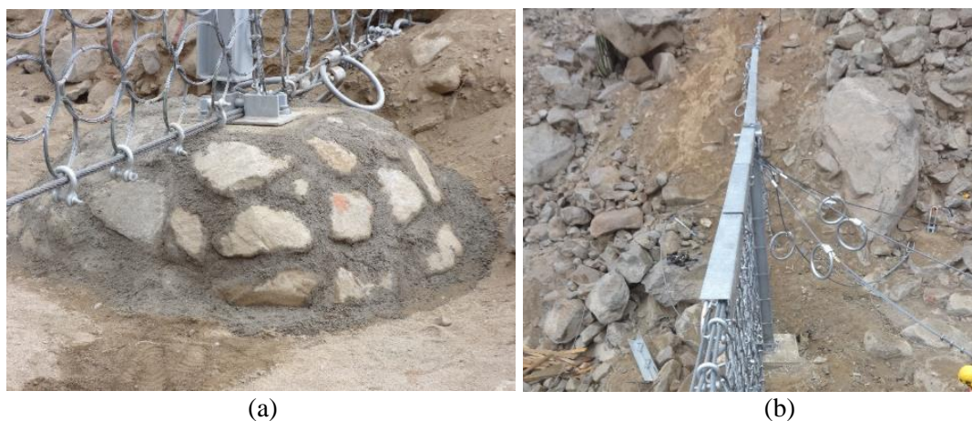
Fig. 6. (a) Scour protection around the posts for UX-barriers; (b) abrasion protection for the top support rope
