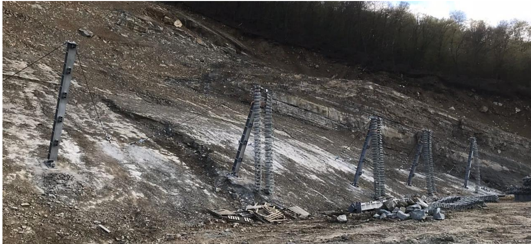
Fig. 7. Ongoing construction in April 2018 of posts for rock fall barrier by Trumer protecting the Samadlo road. Photo: D. Dumbadze
