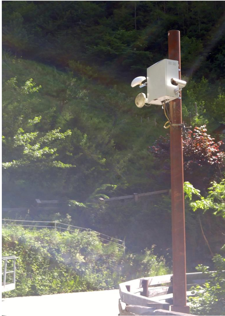
Fig. 4. Radar-System with 2 Radar-Antenna and 1 camera in Lattenbach.
